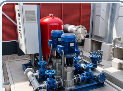
Irrigation Pump Skids
